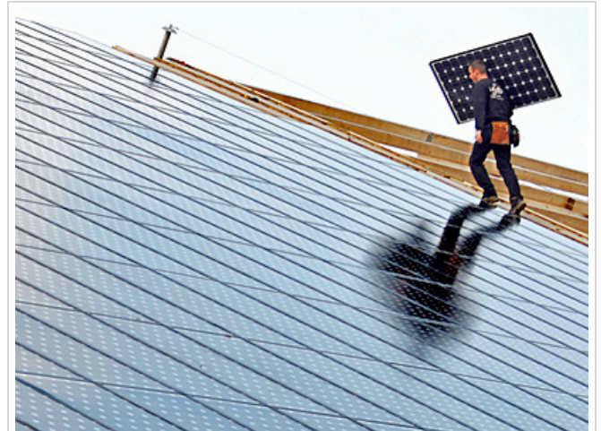
Rooftop solar installations are increasingly common around the world.
